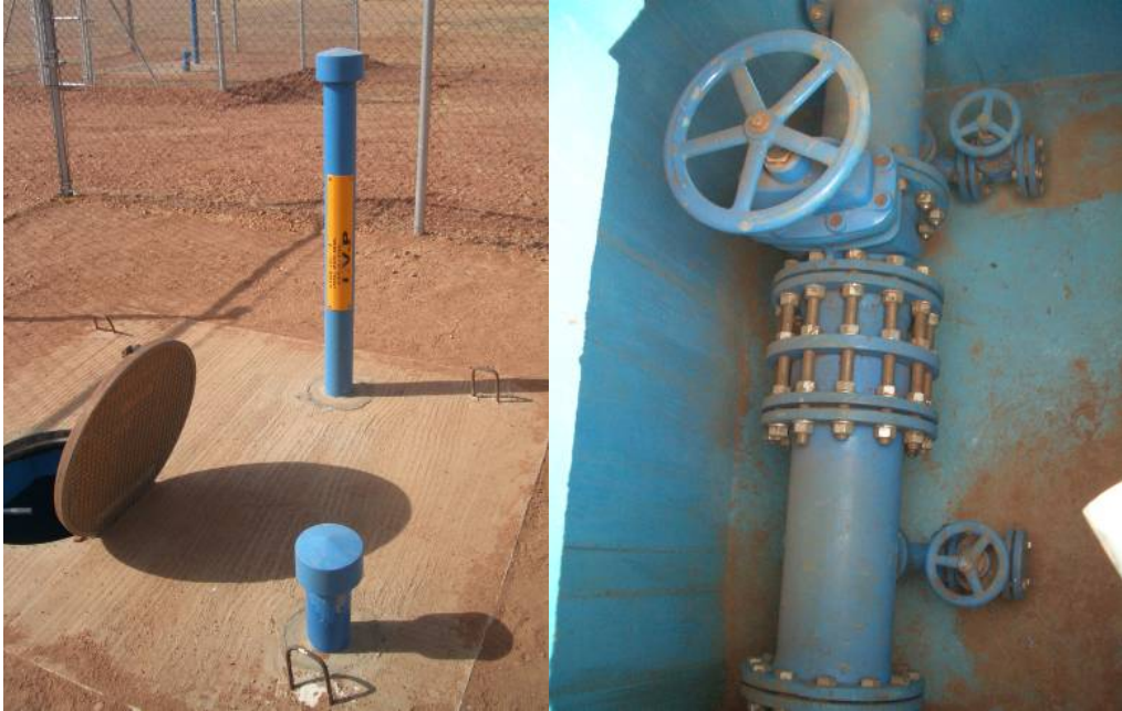
isolation valve chamber interior (c c), pipeline marker post (c r), line vent (d l), fire hydrants (d r)
