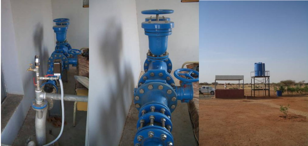
well head (t l, t c) well zone (t r), isolation valve chamber exterior (c l),
